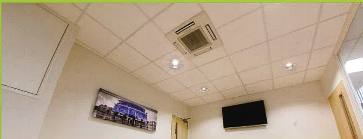
Modern suspended ceilings with energy efficient LED lighting installations and air conditioning systems.
